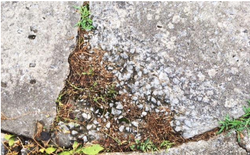
Photos to the left show sidewalk conditions on recent site visit.
