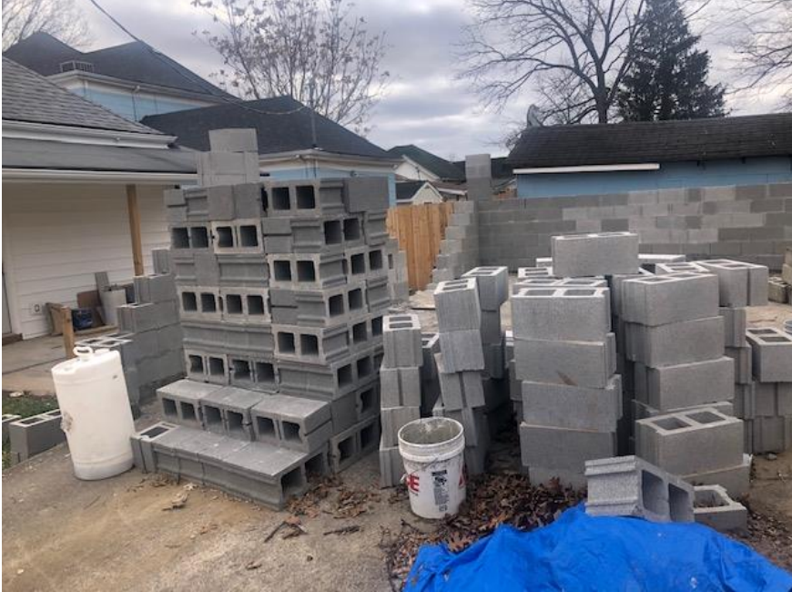
View of partially constructed garage. The primary structure on subject property is located to the left.
