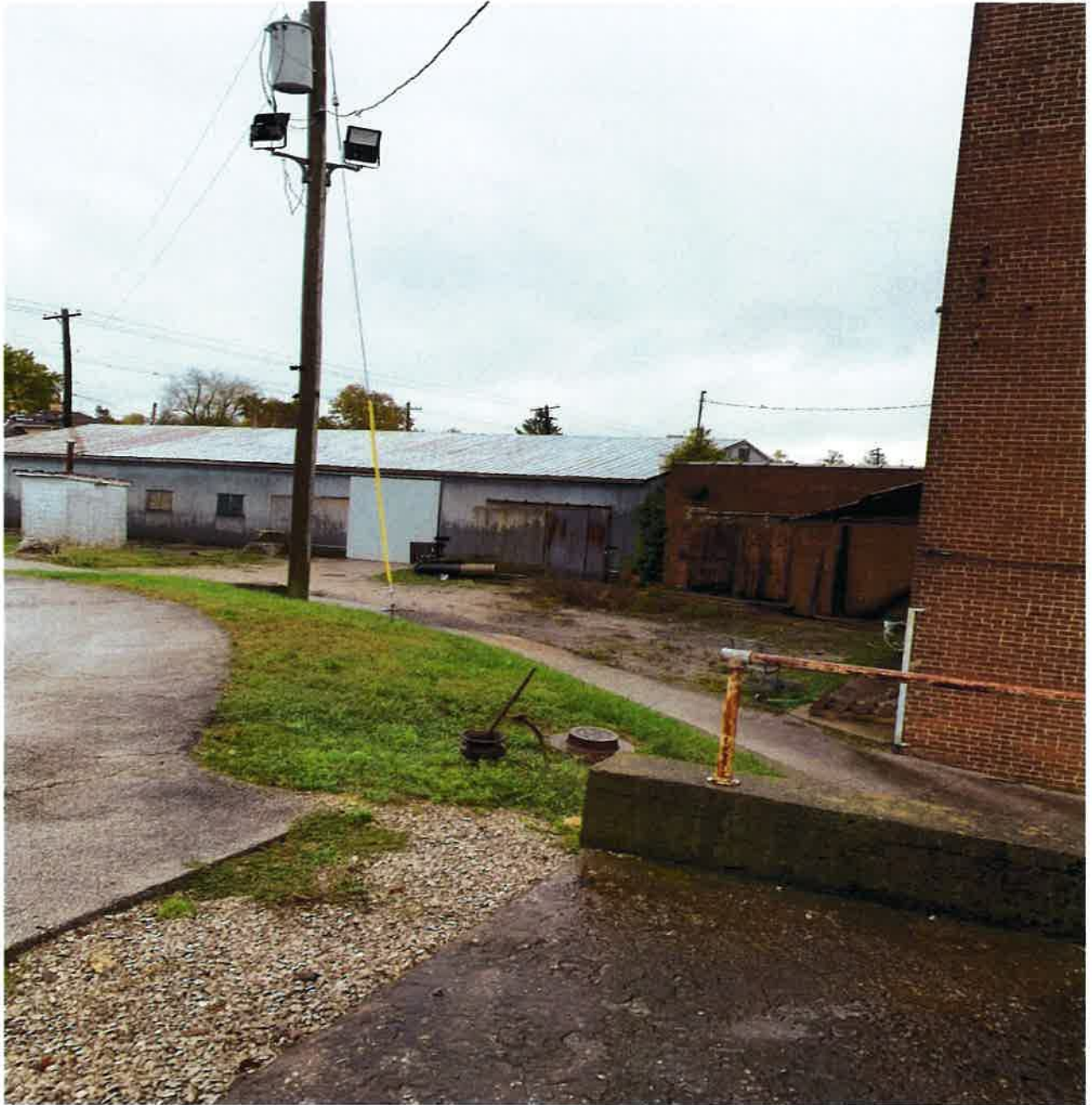
Water meter at northwest corner of Office building
