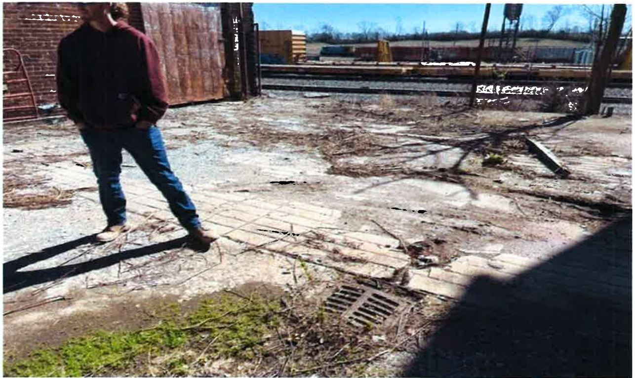
Stormwater inlet between Office building and Annex building
